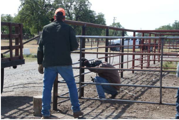
David Brandenberger (kneeling) and Tim Leach work the metal corral fencing. Photo by Roy Stewart
